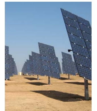
Tracked PV installation (Spain)
